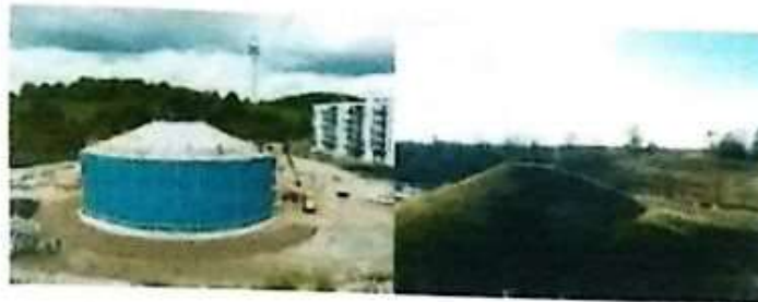
Figure 1 - Large Hot Water Storage (construction and final state) combined with Solar Thermal District Heating "Am Ackermann-bogen" in Munich, Germany
